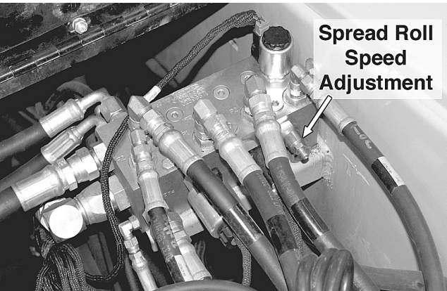
Figure 26. Conveyor/Auger/Spreadroll Manifold Spreadroll Flow Control Valve
